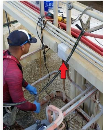
MCOR™ 5511 easily filled in concrete cavities and replicated the beveled feature of the existing concrete.
