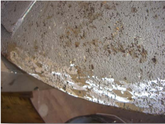
Visible corroded metal confirms harshness of the gas flow
