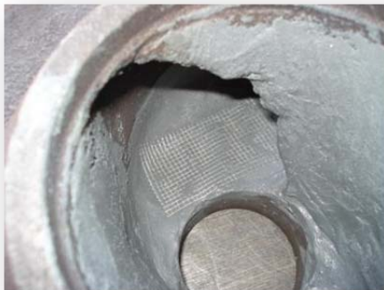
Fabric reinforcement was placed over the holes to provide support and bridge the holes.
